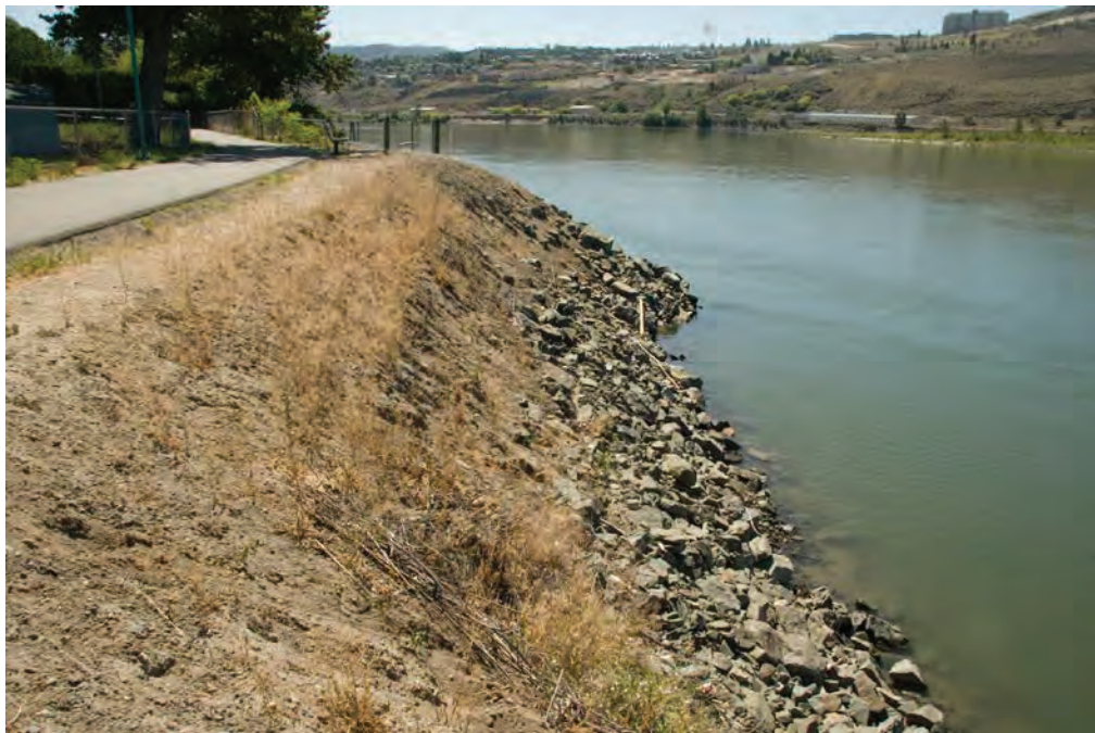
Photo 4. River face of dike behind property showing HWM near top of bare rocks.
