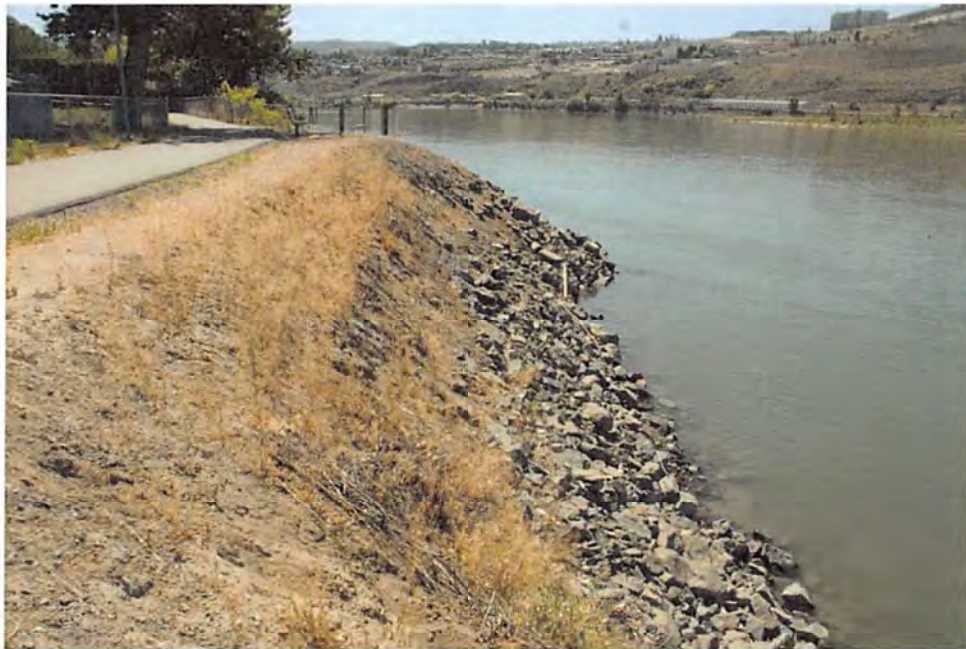
Photo 4. River face of dike behind property showing HWM near top of bare rocks.
