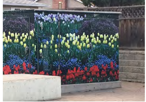
Decorative wrap on an electrical box can help integrate utility installations into landscaped areas
