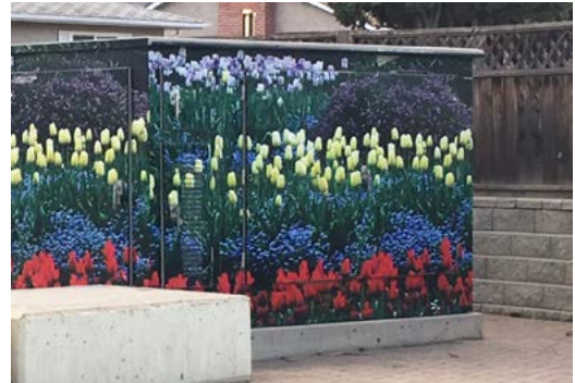
Decorative wrap on an electrical box can help integrate utility installations into landscaped areas
