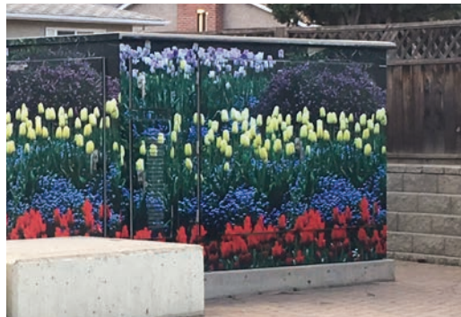
Decorative wrap on an electrical box can help integrate utility installations into landscaped areas
