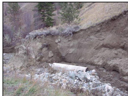
An example of severe creek erosion
