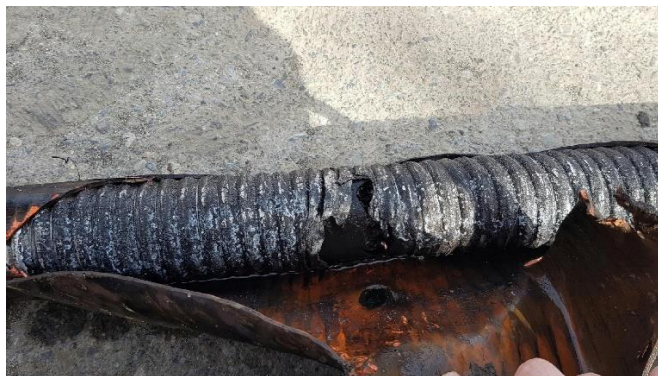
Figure 6: The faulty power line to the KCWQ
