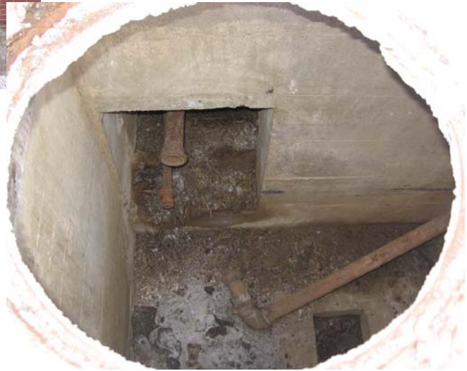
Photo No. 6: Example of manholes outside each bunker providing access to underground piping that ran from boiler to each building. The potential exists for asbestos pipe wrap to still be present below ground (February 4, 2008).
